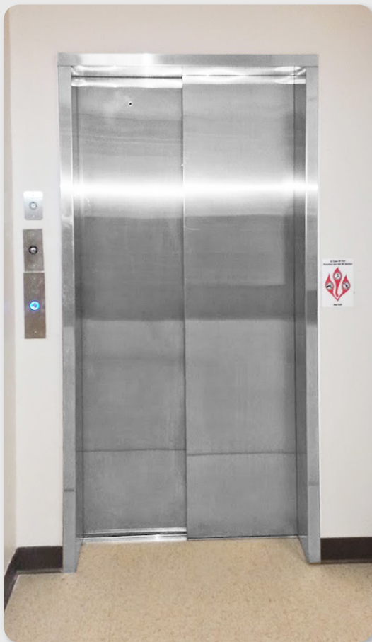
BRUSHED STAINLESS STEEL "ELEVATION" LU/LA ELEVATOR CAR with Brushed Stainless Steel Two Speed Doors.
